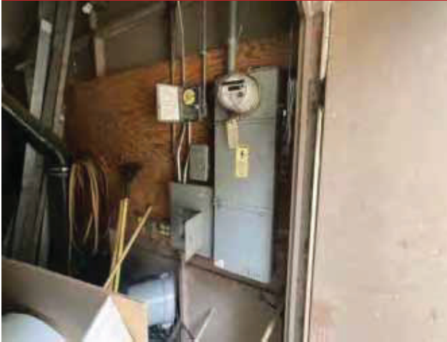
7 - DISTRIBUTION PANEL AND ELECTRIC METER
