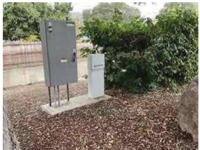
6 - LIGHTING CONTROL AND IRRIGATION PANELS
