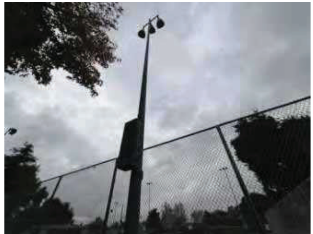
16 - SPORTS COURT LIGHTING
