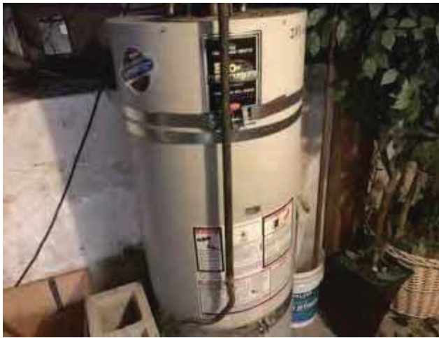
15 - STORAGE TANK WATER HEATER
