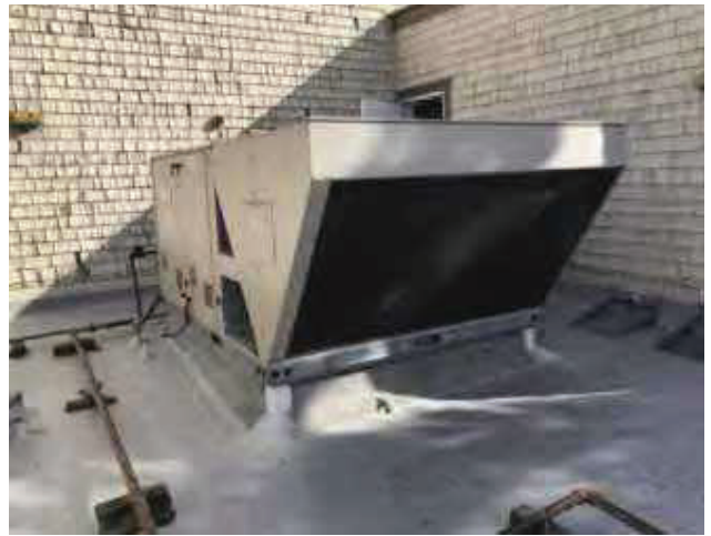
16 - ROOF MOUNTED PACKAGED UNIT
