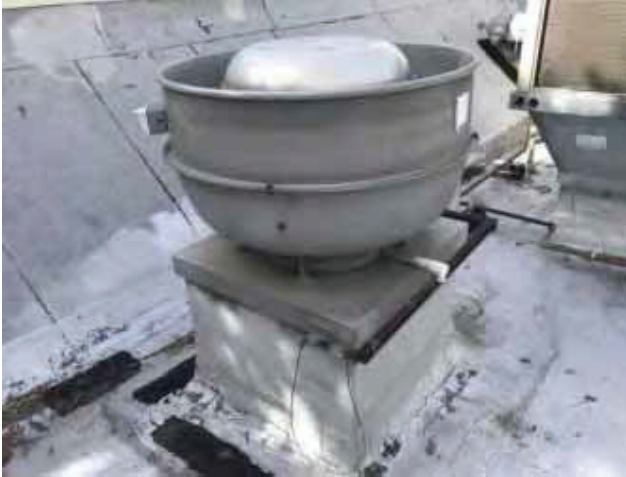
19 - ROOF MOUNTED EXHAUST FAN
