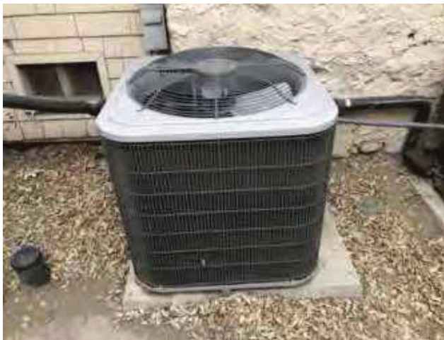
17 - SPLIT SYSTEM CONDENSING UNIT
