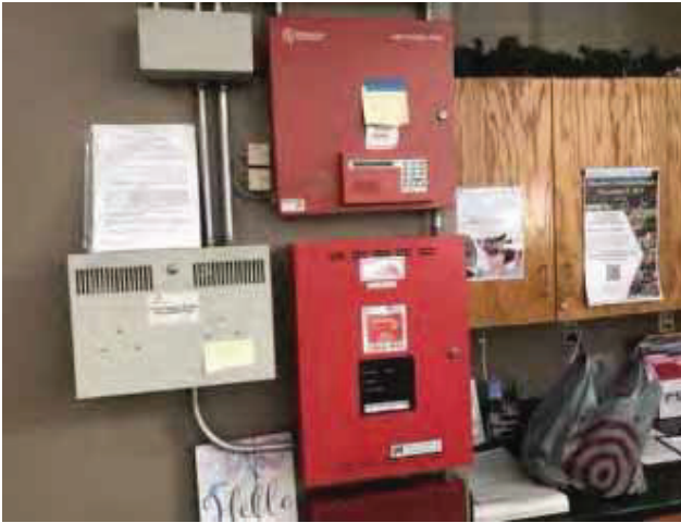
21 - FIRE ALARM CONTROL PANEL
