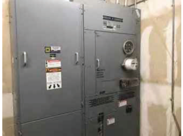
20 - BUILDING MAIN ELECTRICAL SWITCHBOARD
