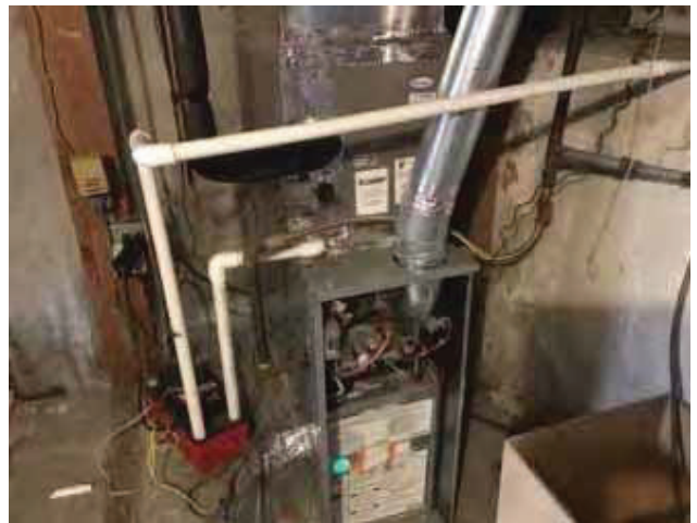
18 - HVAC GAS FIRED FURNACE
