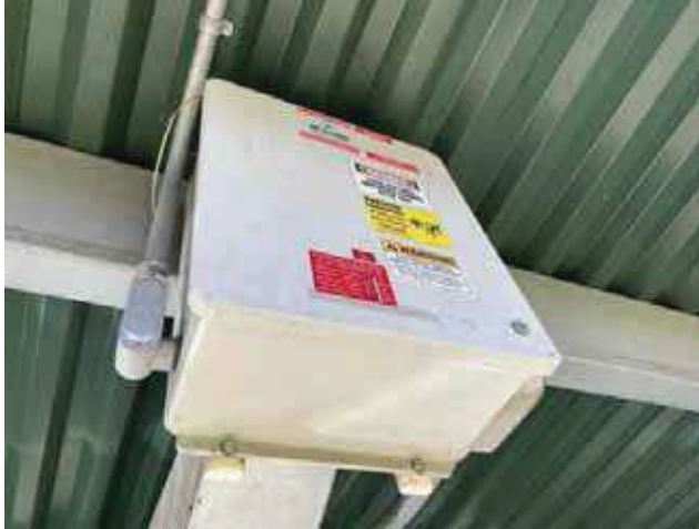
13 - SOLAR POWER INVERTER
