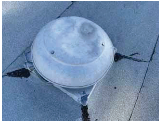
10 - ROOF MOUNTED EXHAUST FAN
