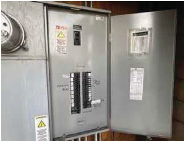
9 - MAIN DISTRIBUTION PANEL
