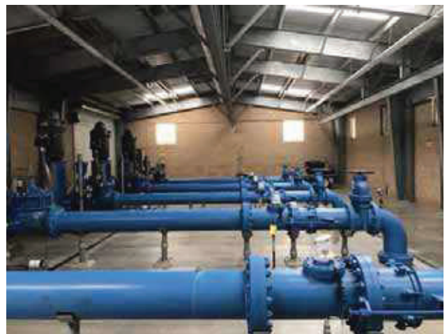
18 - NEW BOOSTER BUILDING INTERIOR
