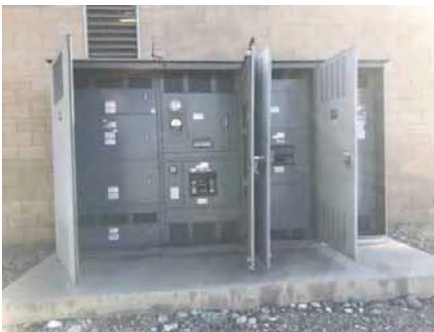
23 - MAIN BUILDING ELECTRICAL SWITCHBOARD
