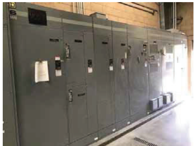
24 - BUILDING MOTOR CONTROL CENTER
