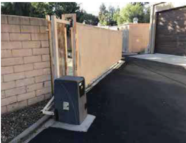
29 - AUTOMATIC GATE WITH CONTROLLER
