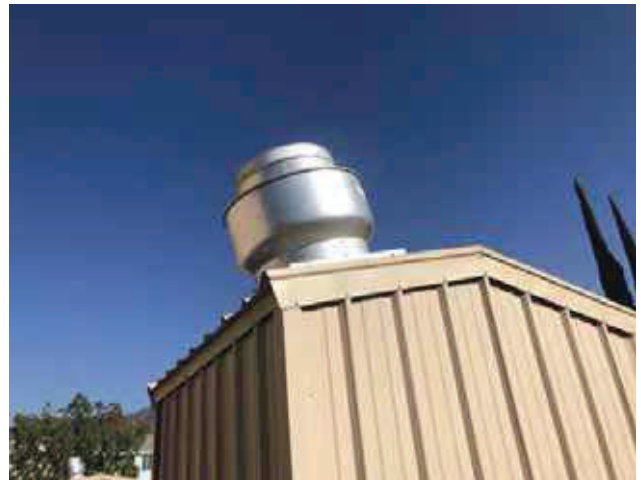
22 - ROOF MOUNTED EXHAUST FAN
