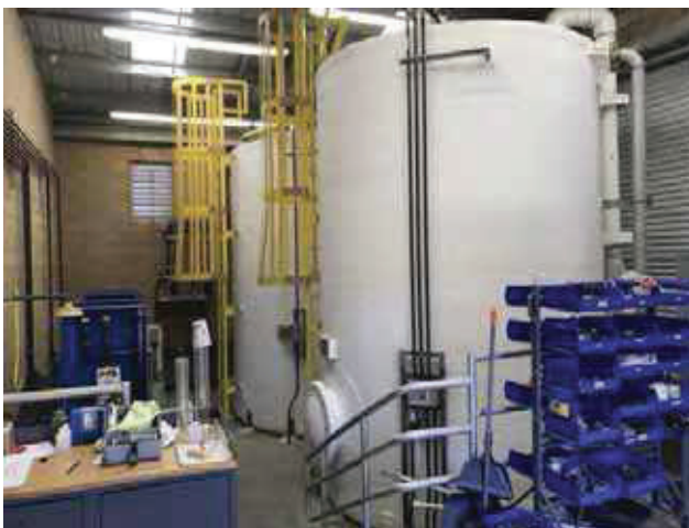
17 - CHLORINE EQUIPMENT INTERIOR AREA
