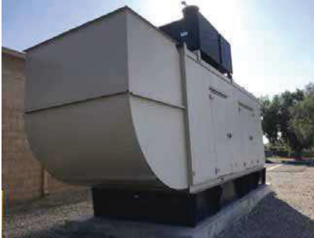
25 - SITE DIESEL EMERGENCY GENERATOR
