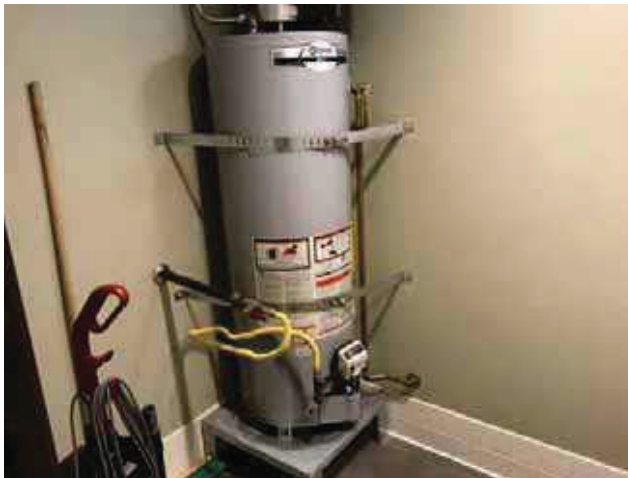
21 - STORAGE TANK WATER HEATER
