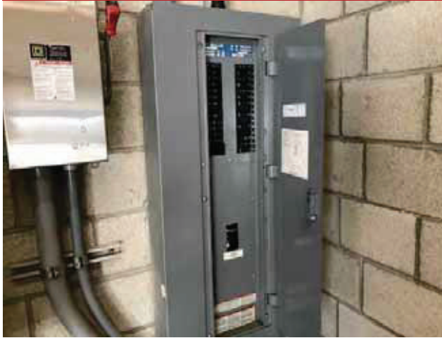
25 - MAIN ELECTRICAL DISTRIBUTION PANEL
