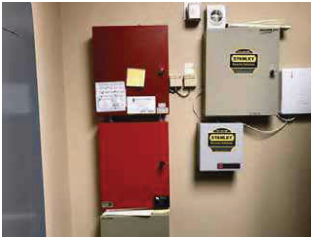
27 - FIRE ALARM CONTROL PANEL
