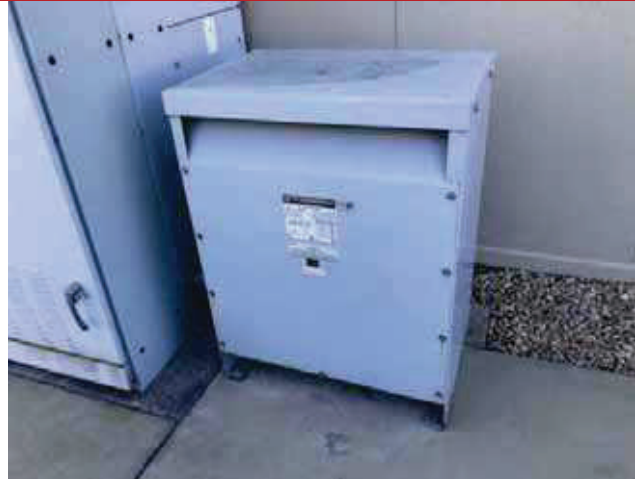
26 - STEP DOWN SECONDARY TRANSFORMER
