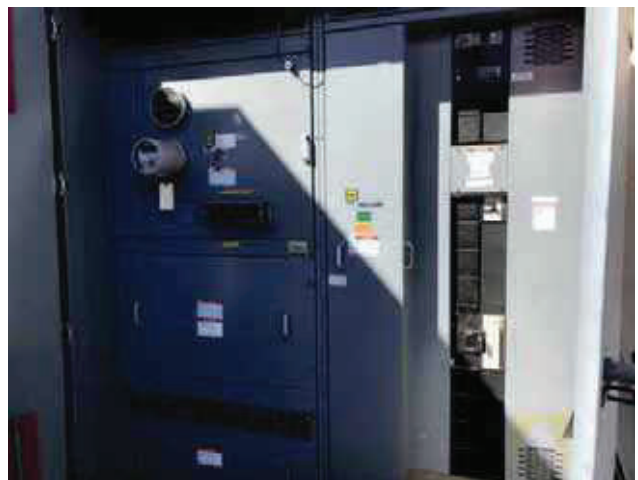
24 - MAIN BUILDING ELECTRICAL SWITCHBOARD
