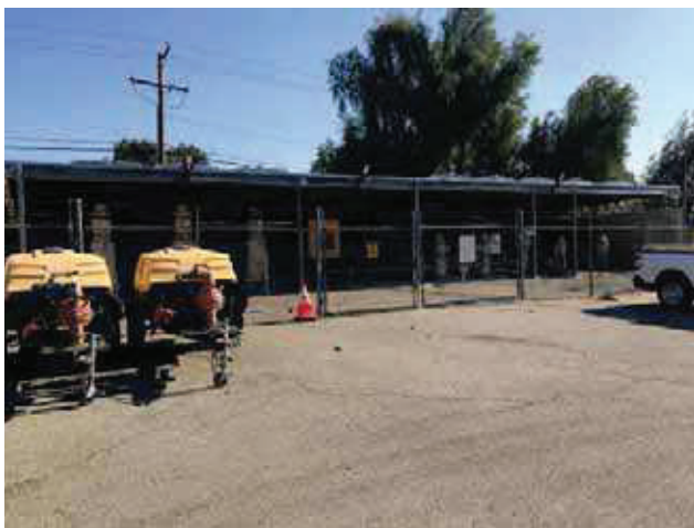
29 - BOOSTER PUMP HOUSING AREA
