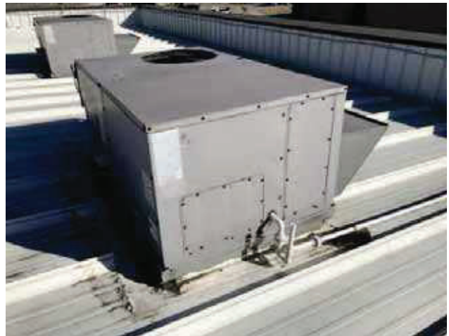
22 - ROOF MOUNTED PACKAGED UNIT
