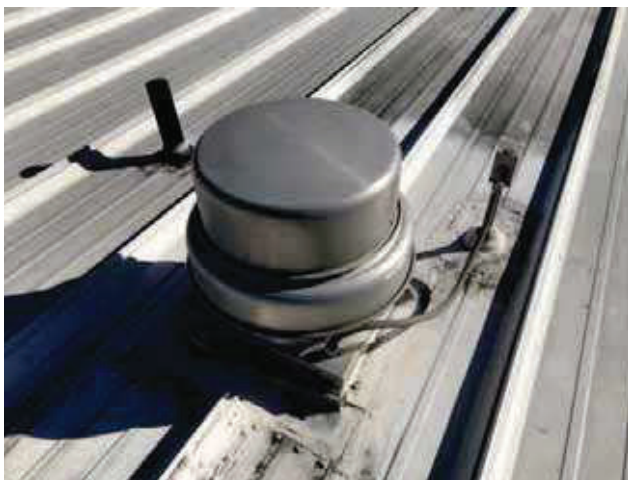
23 - ROOF MOUNTED EXHAUST FAN
